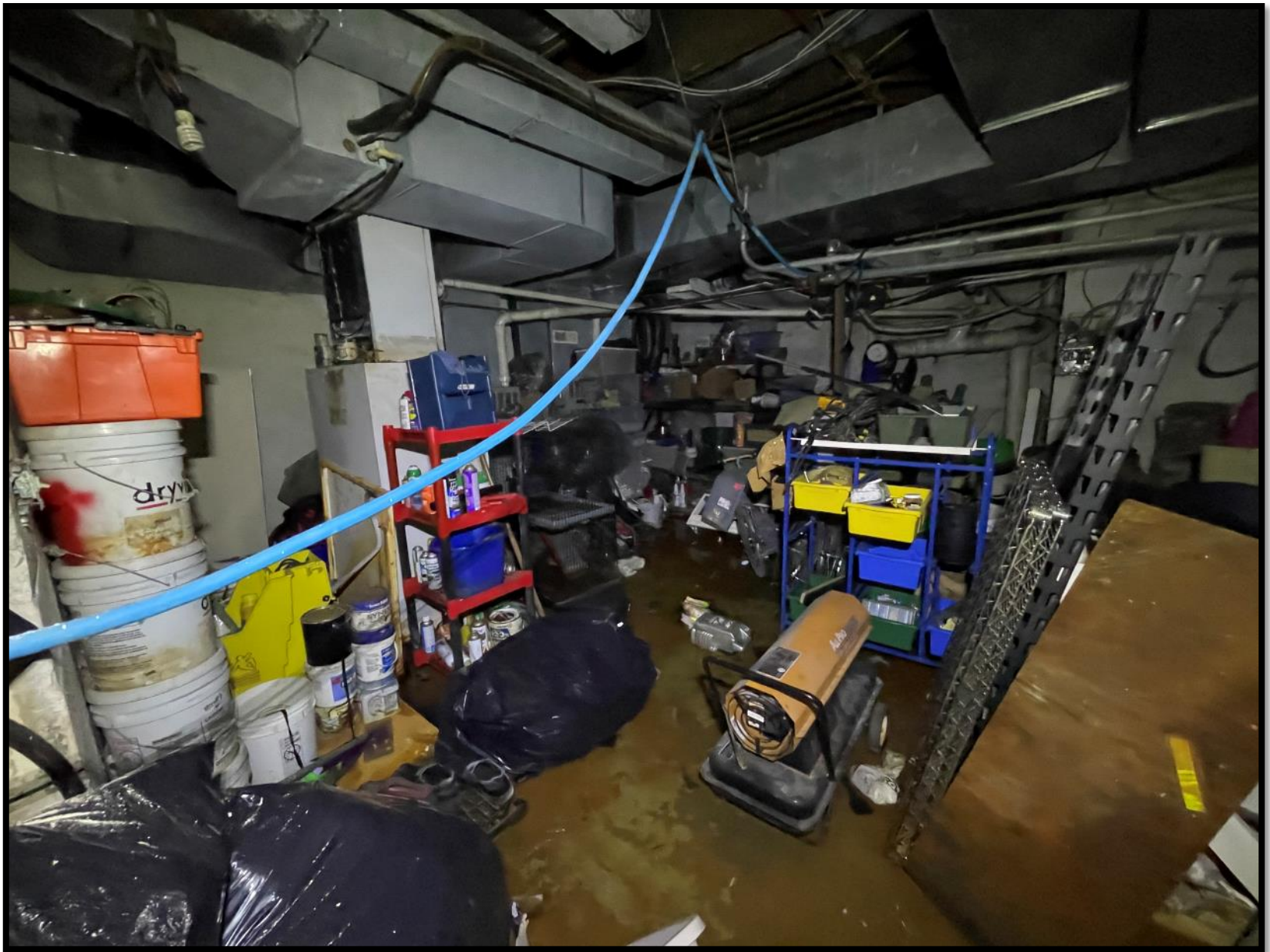
Basement Debris & Water Inundation (Typical)
