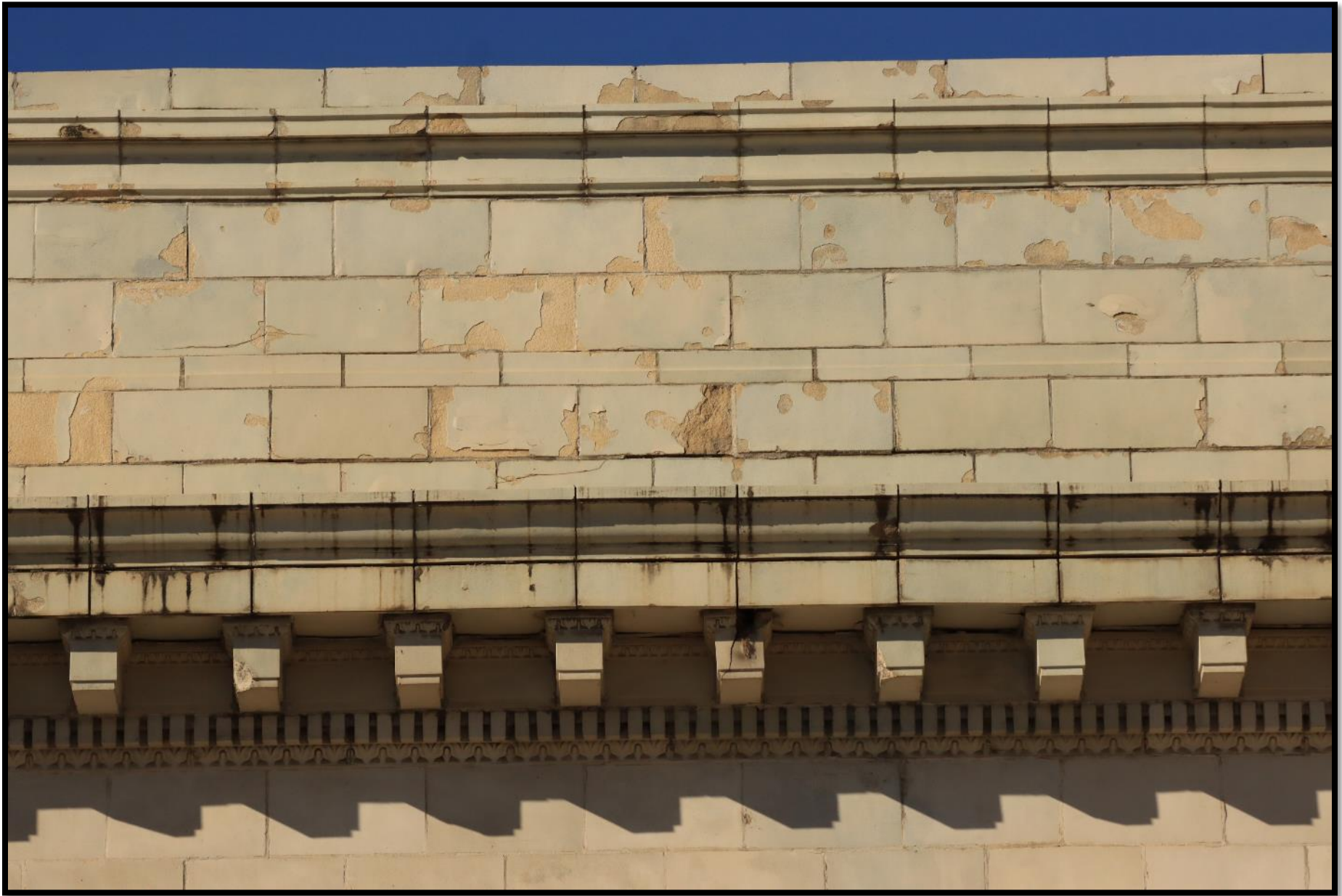
Terra Cotta Spalling (Typical)
